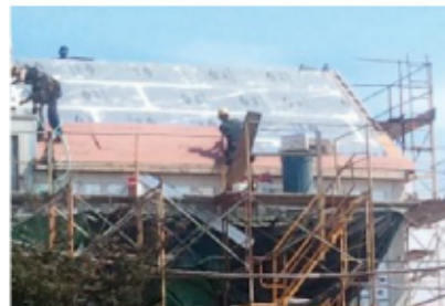
Figure 3. Plywood sheathing, screwed through the foam insulation on the roof and into the rafters, provided continuous nailing for the red cedar roof shingles. The seams were taped per the manufacturer's instructions, and a mesh drainage layer went between the sheathing and the shingles.
